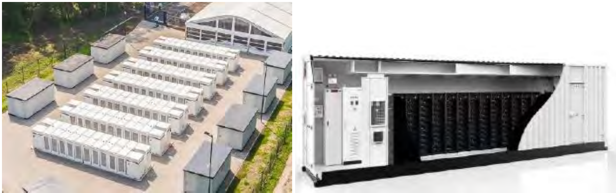
Figure 3.8 Examples of in Prefabricated Enclosures for Battery Energy Storage System Units
