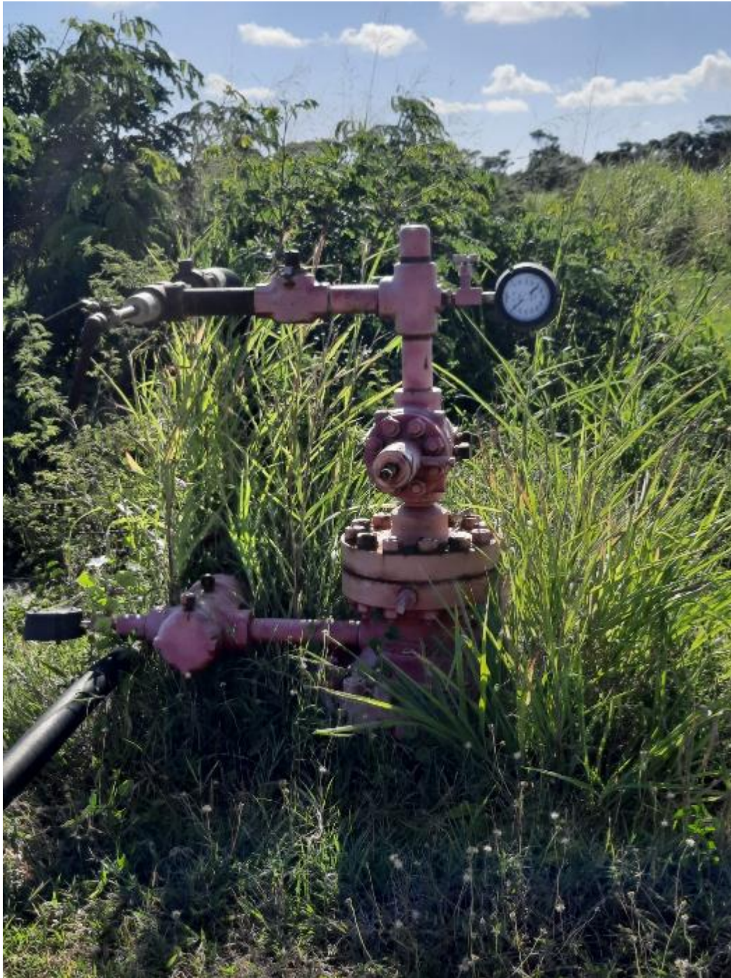
Photo 37 High pressure gas well
