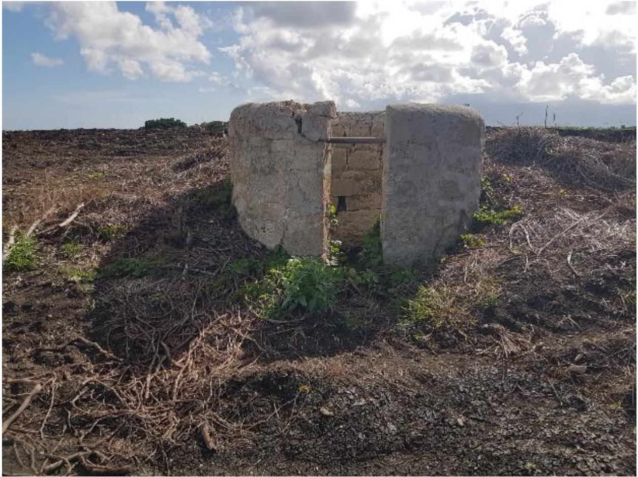
Photo 29 Drainage well A
