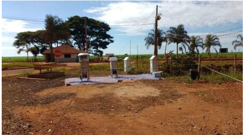
Figure 15 – Overall vision of the equipment at the sampling point.
