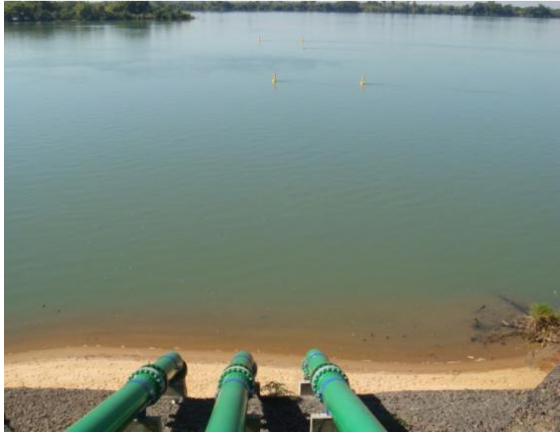
Figure 27 – Effluent discharge. Source: Pöyry, 2018
