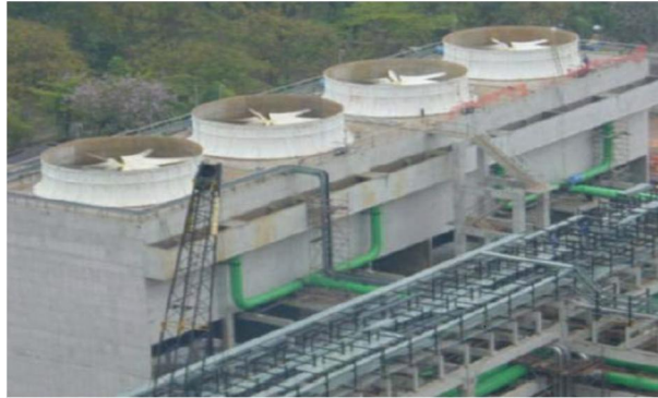
Figure 23 – Cooling Towers. Source: Poyry, 2018
