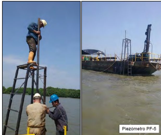
Photo 5.28. Piezometer installed in the sea. Source: EDIFICA COLOMBIA LTDA, in PIO S.A.S (2015) 171
