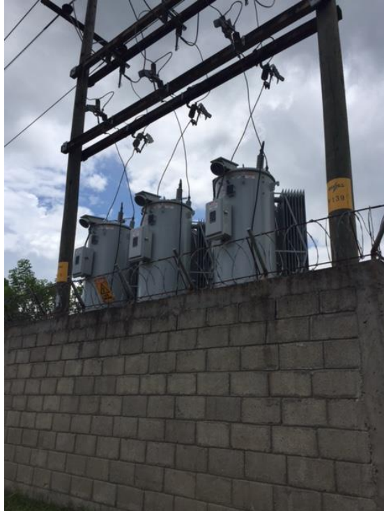
Photo 6 CH Mezapa Power Transformer located in Caserio El Retiro
