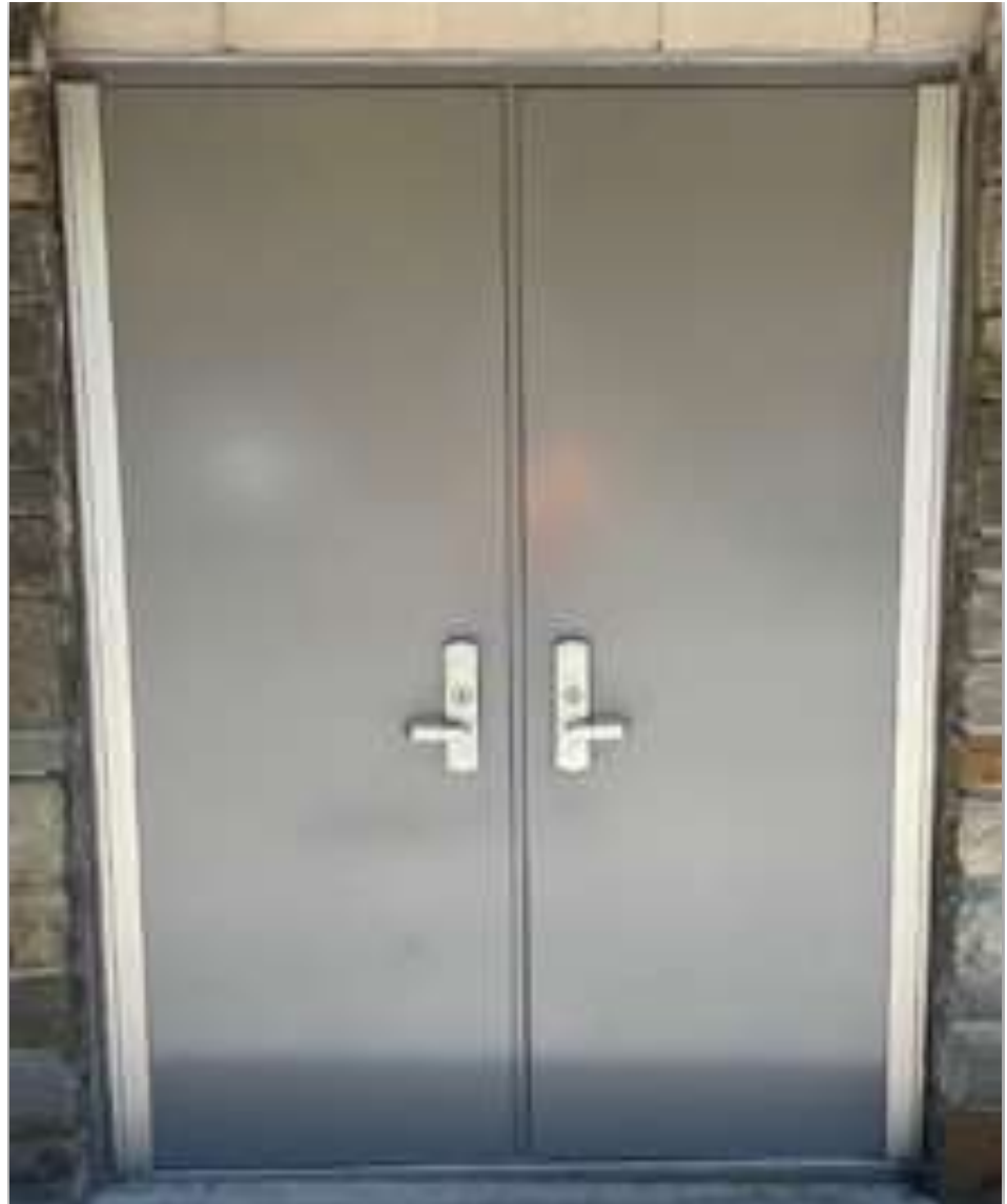
Figure 4.2 Flood door after installation in New York, USA.
