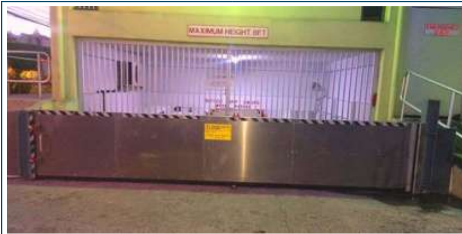
Figure J: Permanent Flood Barrier installed at a SME in Trinidad and Tobago.
