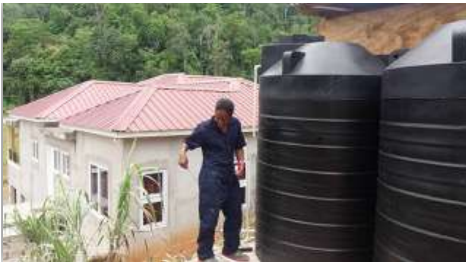
Figure 4.19 Example of water storage tank
