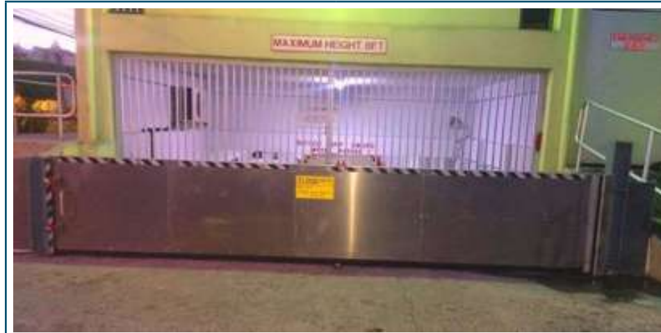
Figure K: Permanent Flood Barrier installed at a SME in Trinidad and Tobago.
