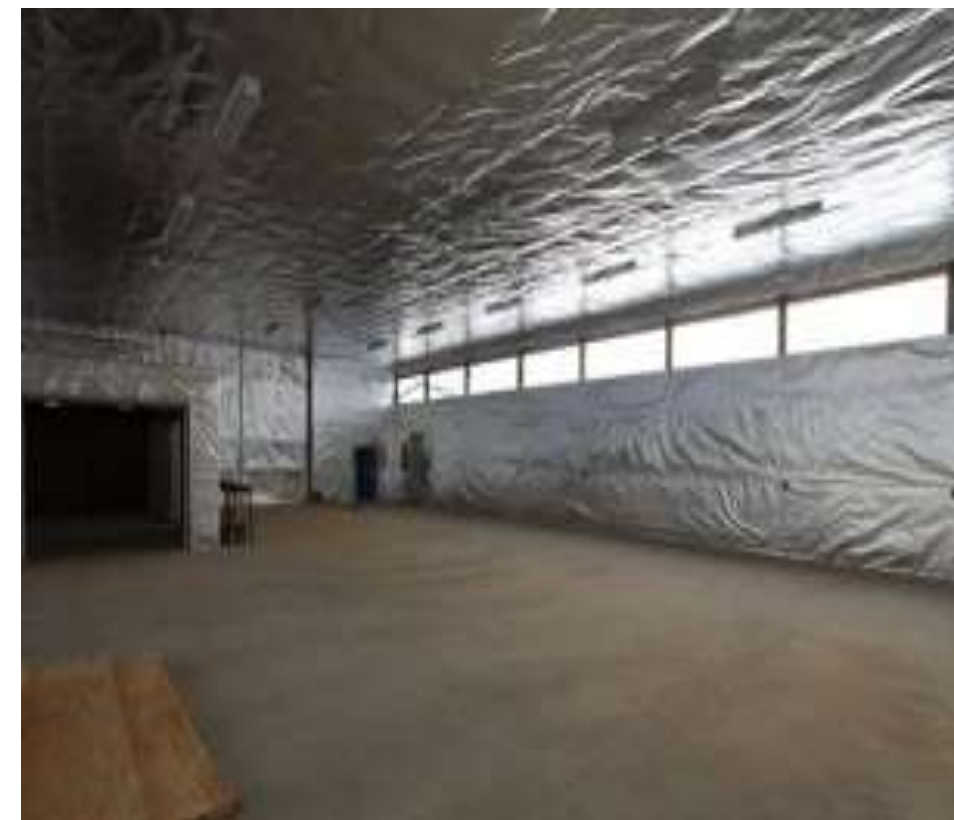
Install a 10mm layer of Prodex (radiant barrier and 10mm insulation) to exterior walls (SMEs)
