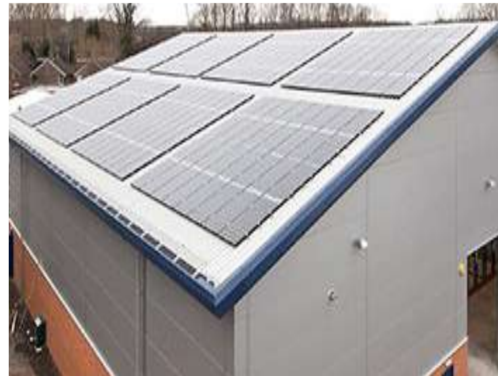
Installing a 60 KW photovoltaic system on the sheet metal roof to generate renewable electricity; absorb and emit solar heat.
