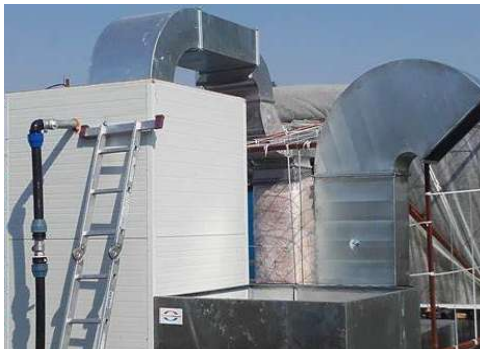
Figure 4.17 Examples of installation of Recycling water from AC units
