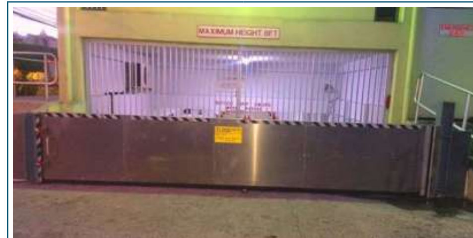
Figure J: Permanent Flood Barrier installed at a SME in Trinidad and Tobago.
