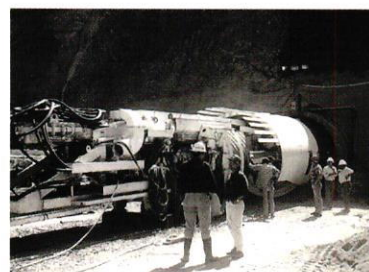
State-of-the-art tunnel-boring machine used by a Venezuelan contractor during construction of the Hidroeléctrica Río Las Vacas power plant in Guatemala
